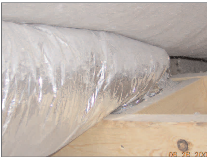
Duct constricted by bend into boot
