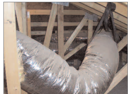
Improper duct support and excess duct sag
