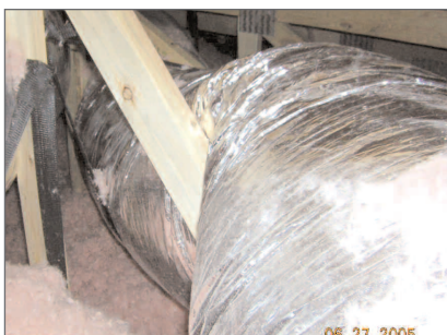
Duct constricted by bend over truss web
