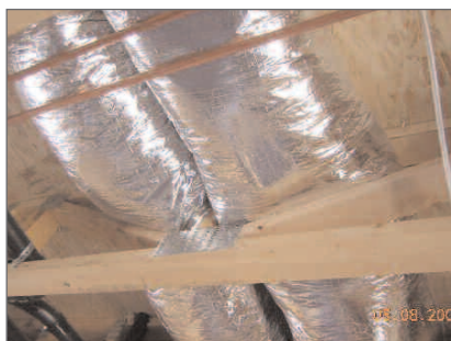
Ducts compressed into small space
