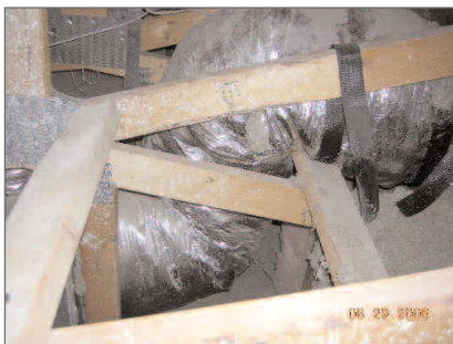
Duct constricted by two bends leaving plenum
