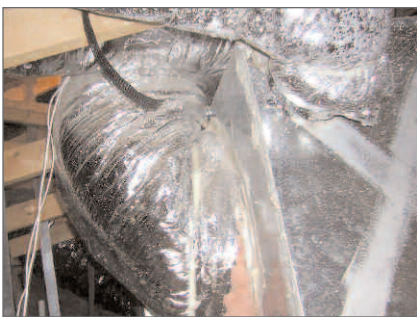
Duct constricted by bend leaving plenum
