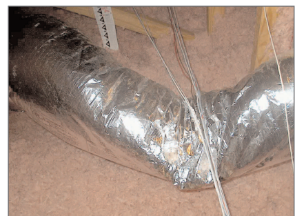
Duct compressed by wires
