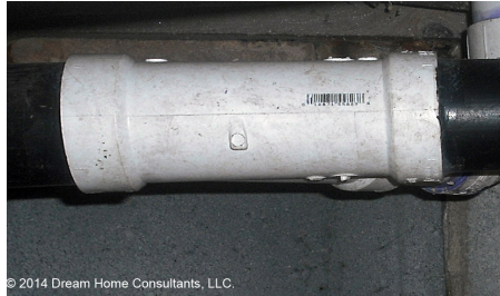
Most solvent cement connections between ABS and PVC are wrong.
